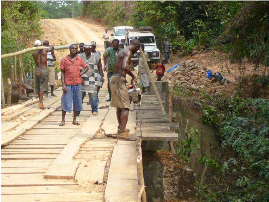
Paramount Chief Jibilla and SLRA Maintenance Director Gbembo (in the green shirt) watch the start phase of putting in a new bridge.
