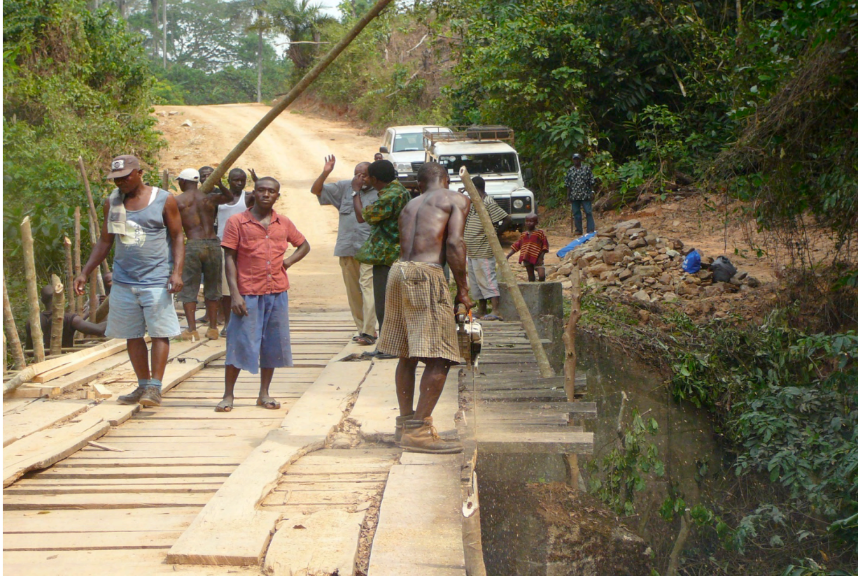
The SLRA workers begin to take down the Sengema Bridge. The long poles being installed are the scaffolding that will support the framework to be built for the bed of the new concrete bridge.
