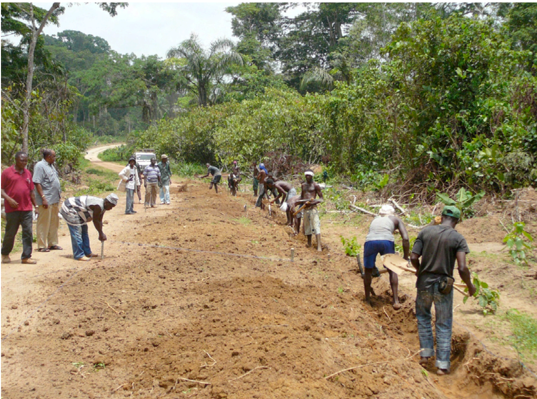
The Paramount Chief marking one side of the road while the men ditch the other side leading to Sengema Bridge.
