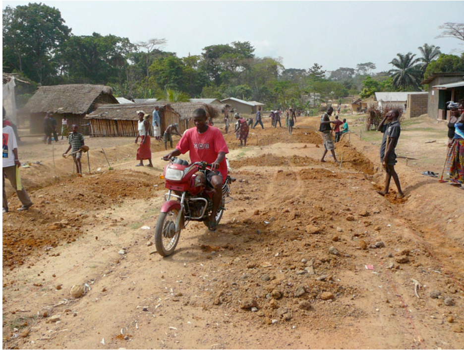
As we arrive in Sandaru late on March 19, we see the people making a difference by ditching the road through the town.
